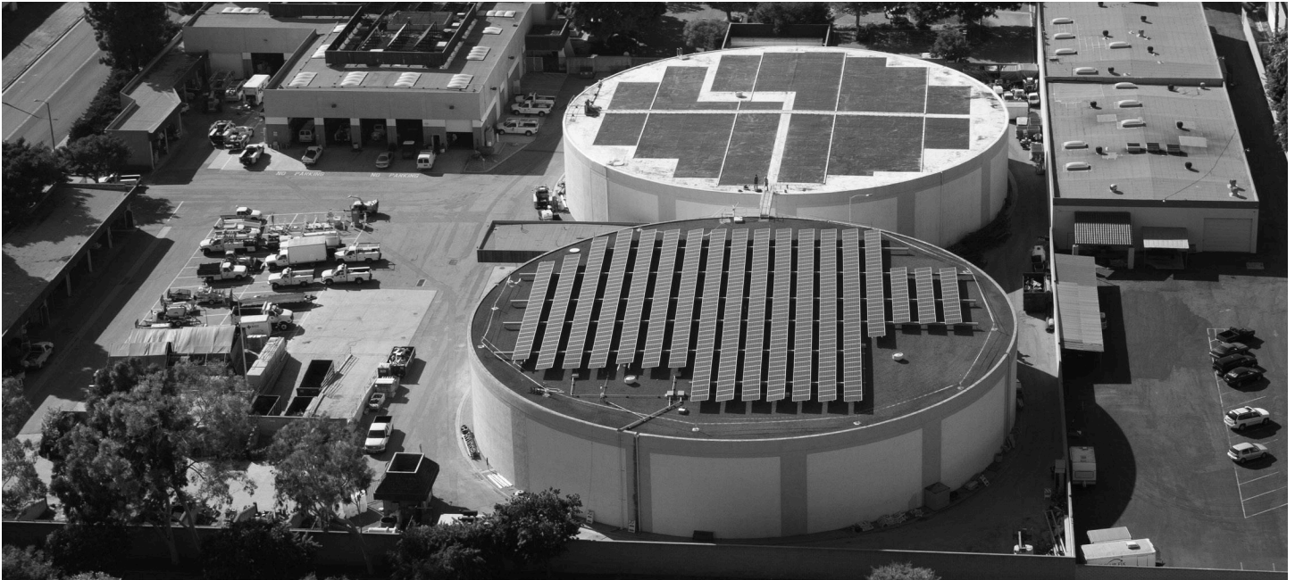
Water Storage with Solar Panels, City of Cerritos Corporate Yard
